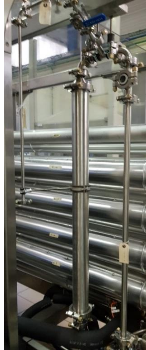
Figure 8 – Oscillator Protection Loop Installed on a NiTech DN43 COBR
